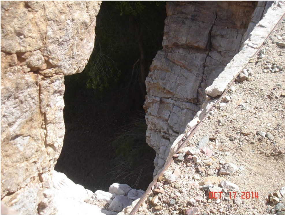
Looking down over an old dam in a canyon on the Ripsy Mine trail
